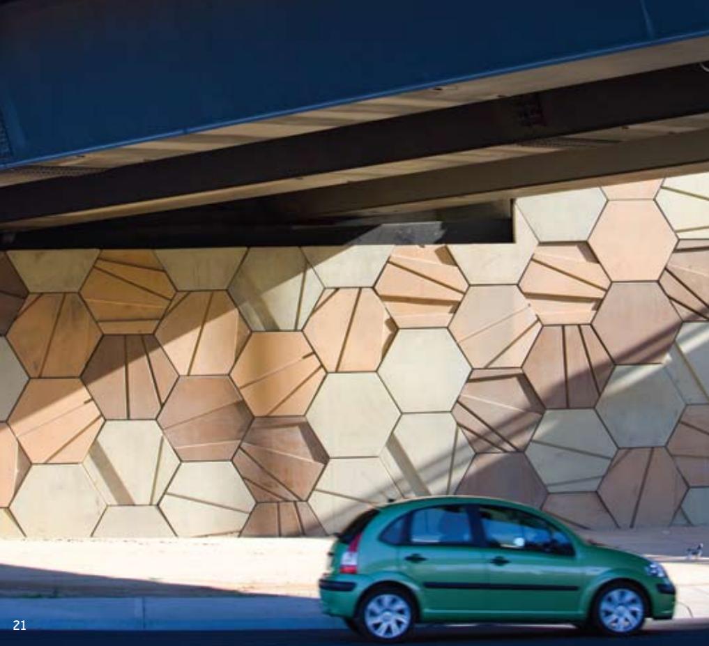
No 21 Facing panels for reinforced earth cuttings were designed to echo the colours of the ground
