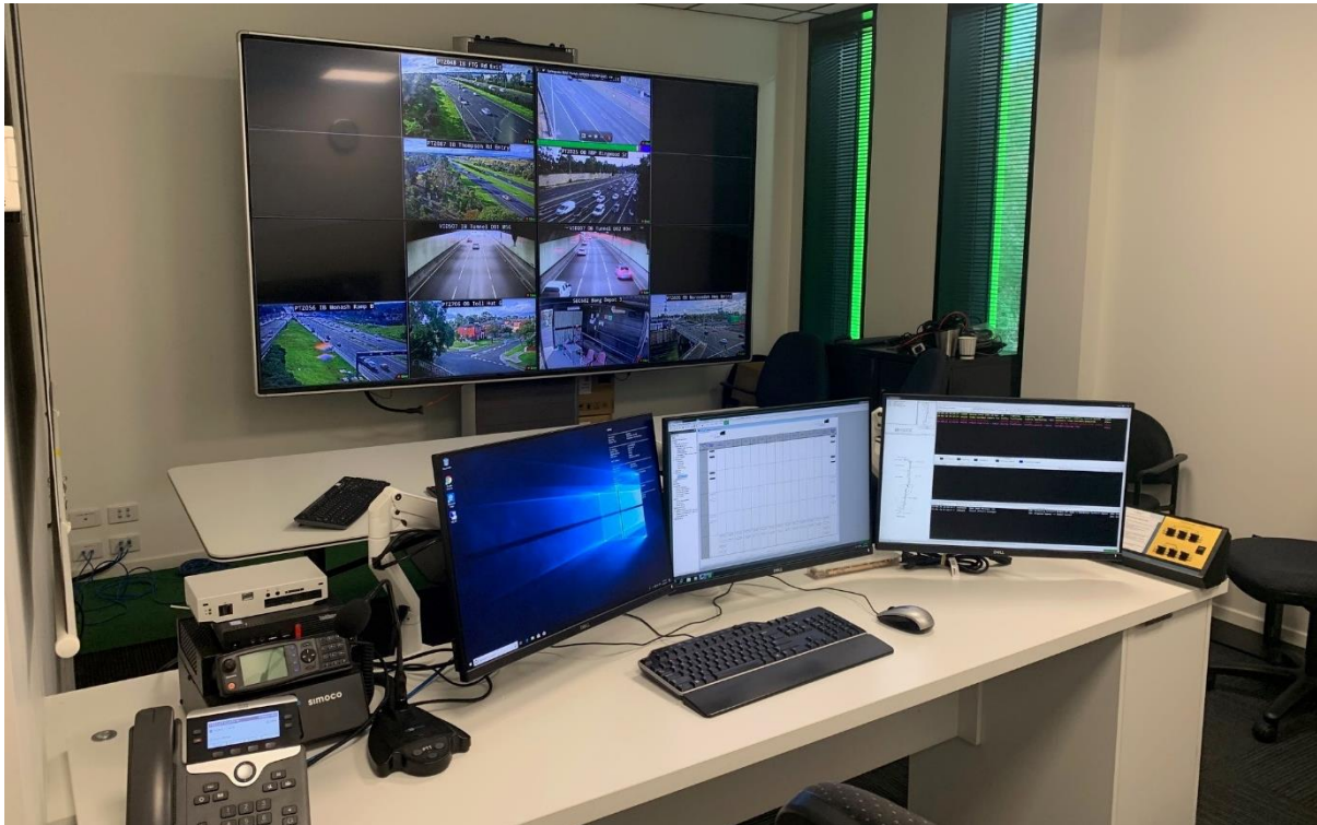
Image 3: A part of EastLink’s back up traffic control room nearing completion
