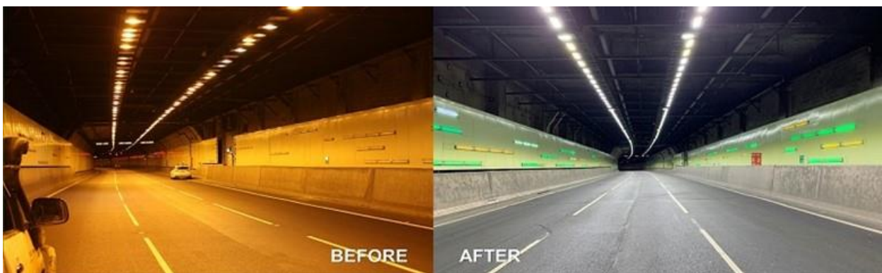
Image 4: EastLink tunnel lighting is now brighter and whiter than before
