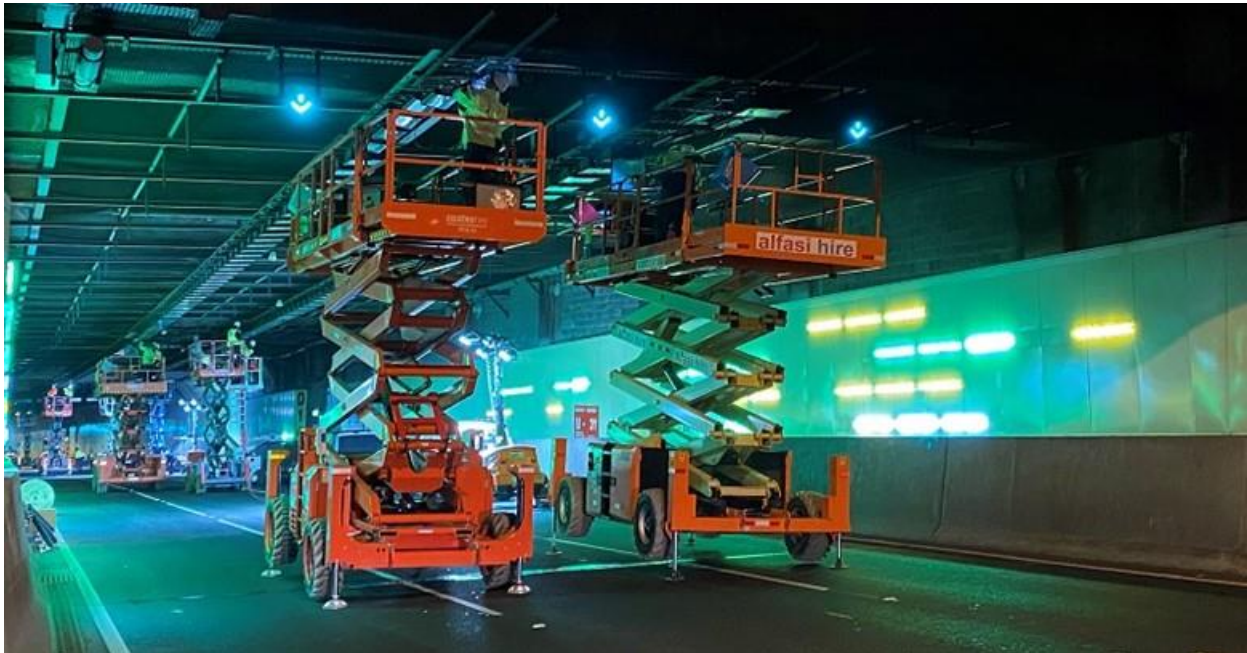
Image 16: Up to 60 technicians and 22 scissor lifts worked over four nights to install 1,174 new LED lights
