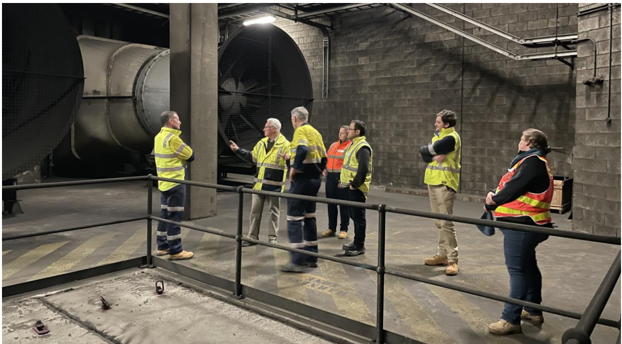
Image 20: Stakeholder tour for Ventia and Department of Transport in the tunnel ventilation facility (22 May 2021)
