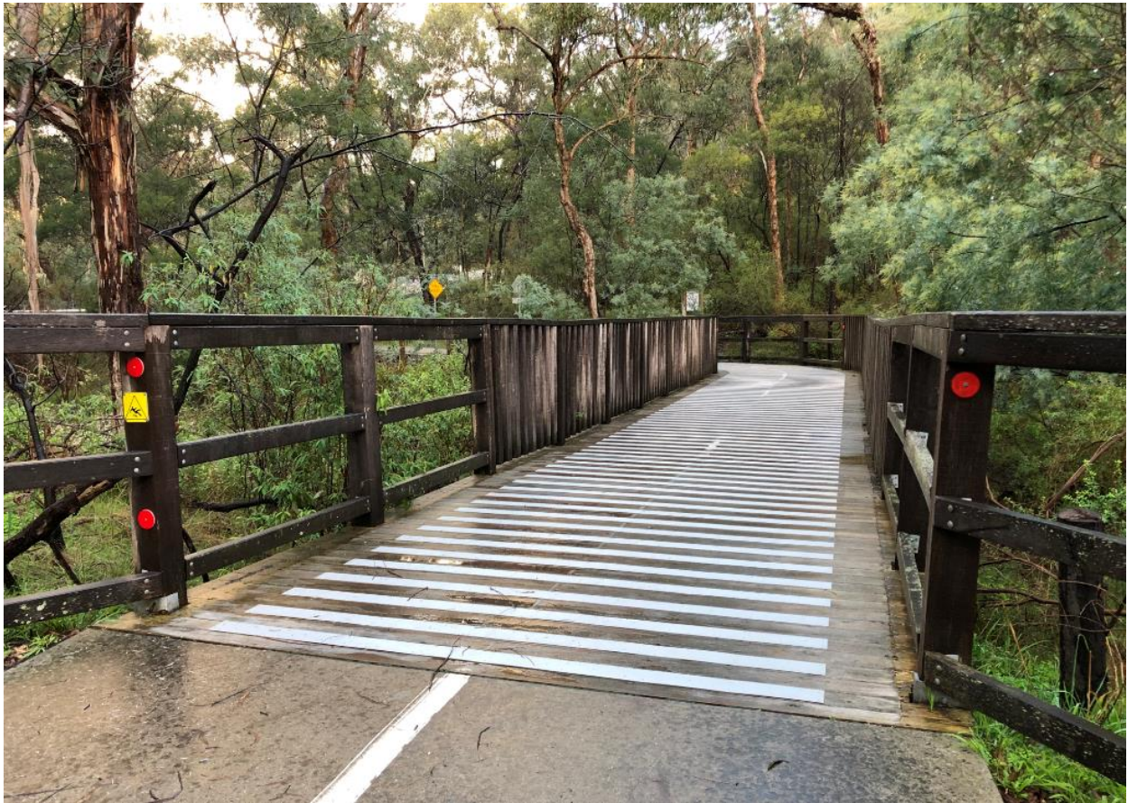
Image 5: New anti-slip strips on a timber bridge on the EastLink Trail in the Mullum Mullum park.
