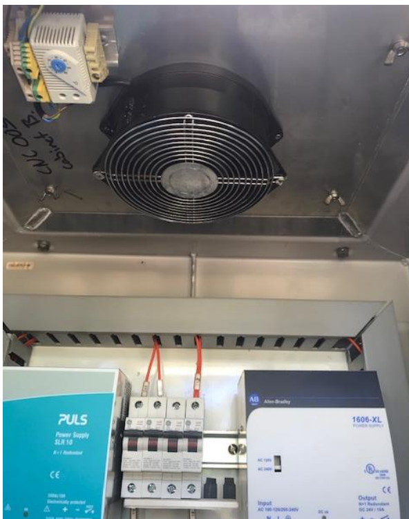
Image 47: Example of an upgraded cooling system installed in one of EastLink's roadside cabinets
